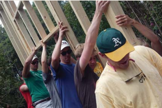
Scholars from the class of 2015 help position a wall during the service project with Albemarle Housing improvement program.
